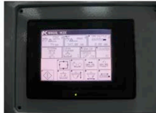
PLC Touch Screen Control
